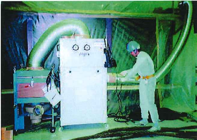
Ventilation device for blast working (It collects blast dust effectively.)
